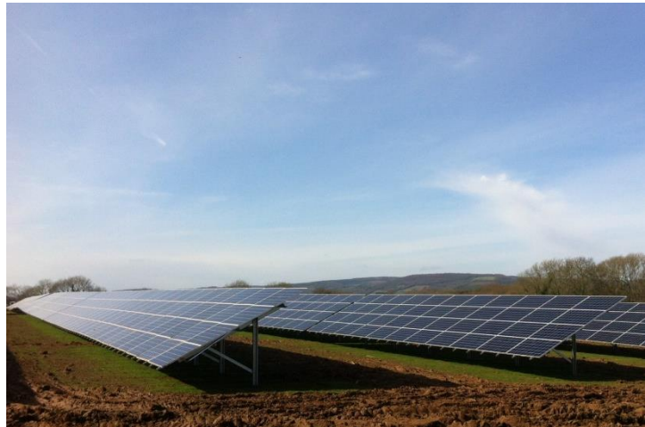
Figure 26 - Oak Grove Solar Farm
